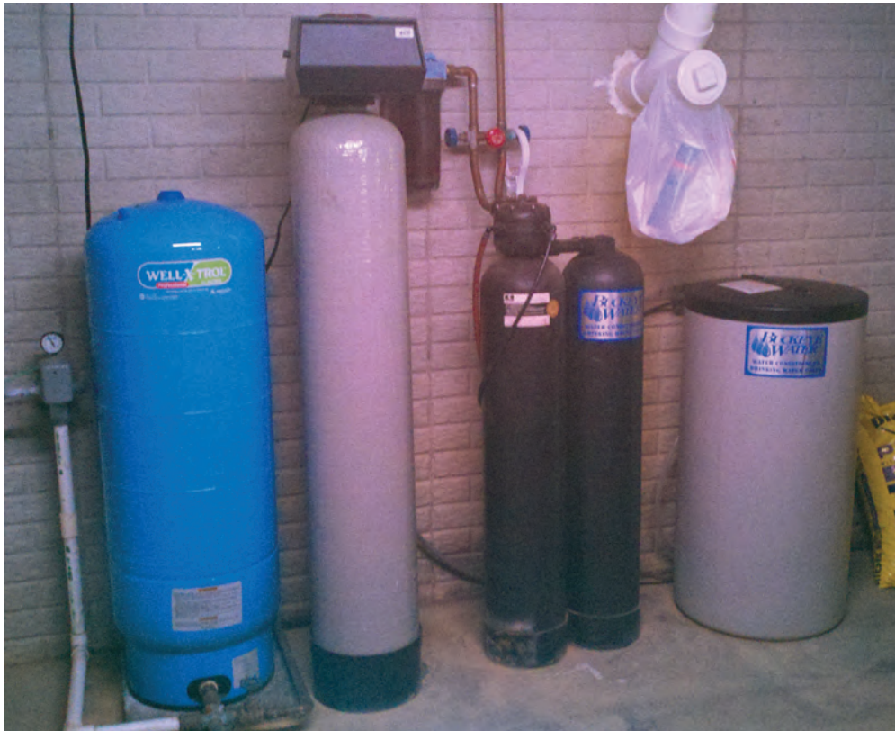
Oxidation/filtration is typically part of a whole-house treatment system installed in the basement of a home. Photograph by Mike Ekberg, Miami Conservancy District.
