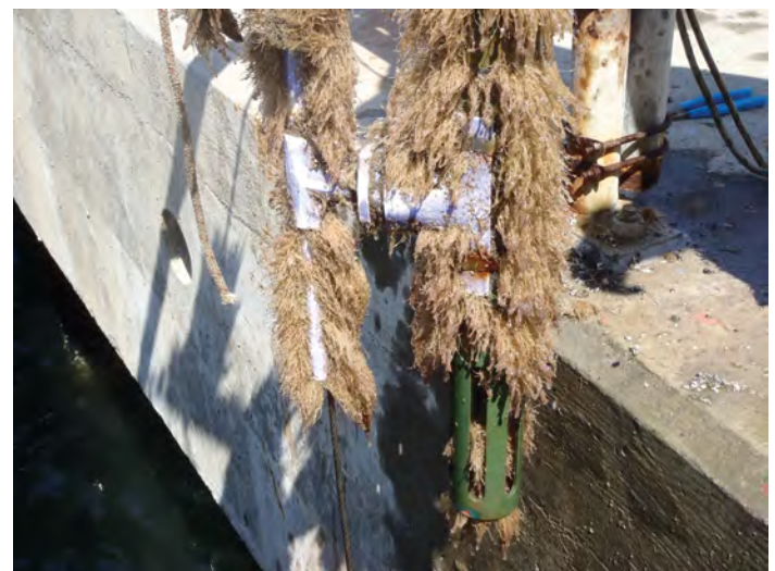
Figure 5. Biological fouling on water-quality instruments at the Richmond-San Rafael Bridge.
